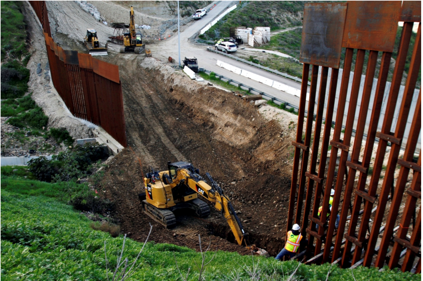
Construction workers in the U.S. work on a new section of the border wall as seen from Tijuana, Mexico, Feb.18. (CNS/Reuters/Jorge Duenes)
