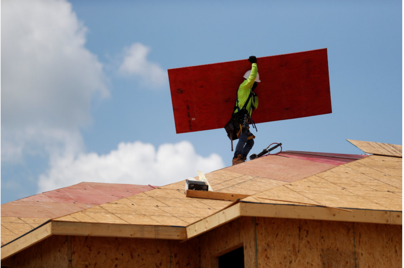
A carpenter works on building new townhomes in Tampa, Fla., May 5, 2021. (CNS/Reuters/Octavio Jones)
