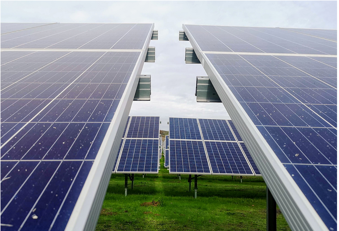
Rows of solar panels on a solar farm (Unsplash/Creative Commons/Mariana Proença)
